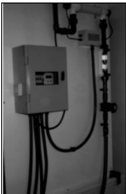
Panel and equipment at back of system
