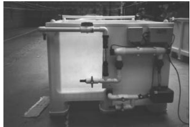
Panel mounted seawater recirculation equipment
