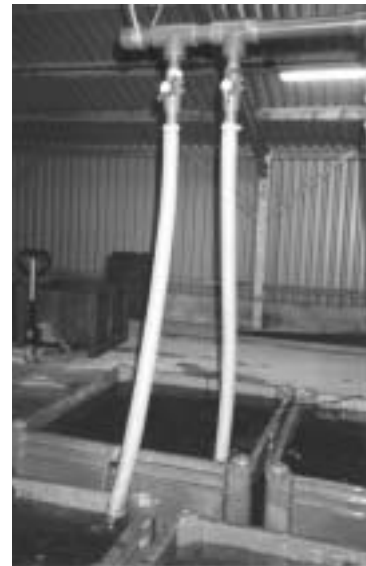
Flexible feed pipes and control valves
