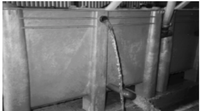
Seawater outlet pipes
